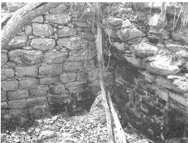
Fig. 13. Remaining part of the vault in Room 2, Structure 2. Please also notice the niche in the walled part between the western doorway column and the western doorjamb in the lower right corner of the picture. Photo: Eduardo González Arce, 2015.
