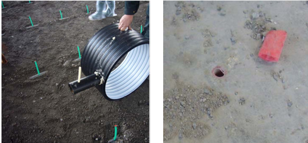
Figure 2. Tube system for aeration of the CBP. The picture to the left shows the vertical tubes before laying the concrete floor, and an illustration of the junctions of the three tube types. The picture to the right shows a vertical tube cut off at the height of the finished floor.
