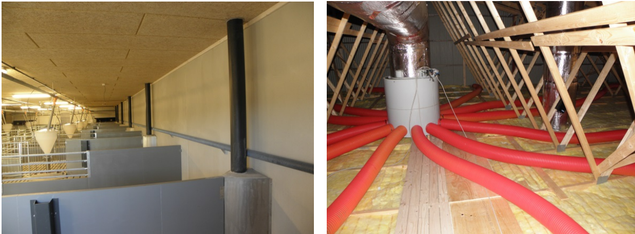
Figure 4. Pit exhaust suction tubes between each second pen (to the left) and combining of twelve pit exhaust suction tubes to a single exhaust in the attic (to the right).
