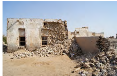
Al Jumail, S54, stonework with mud mortar and cement plastering. Anhydrite plaster finish on the façades, no anhydrite finish on the courtyard wall (right)
