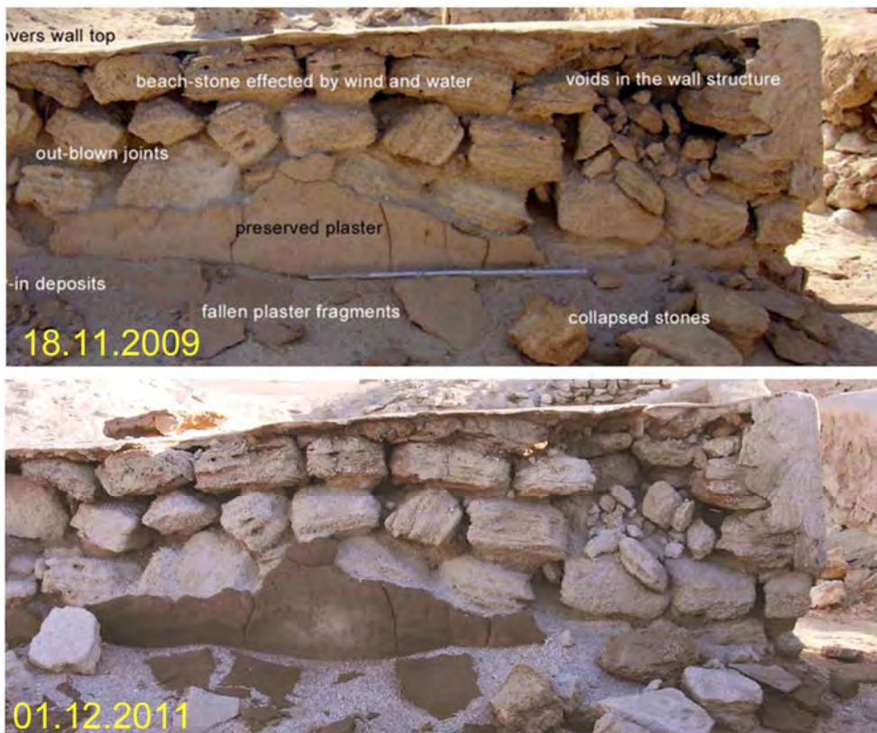
Figure 35: Loss of wall plaster at wall c, room 006, South Field
