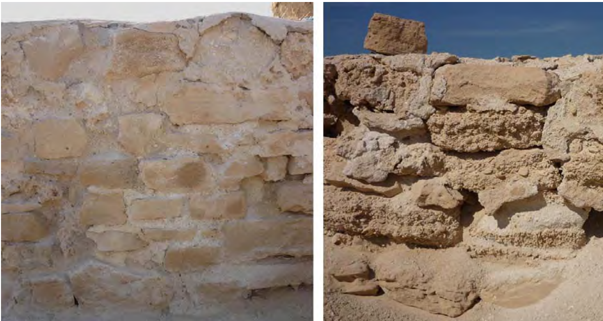
Figure 1: Preservation state of wall structures as a function of mortar and rock stability.
