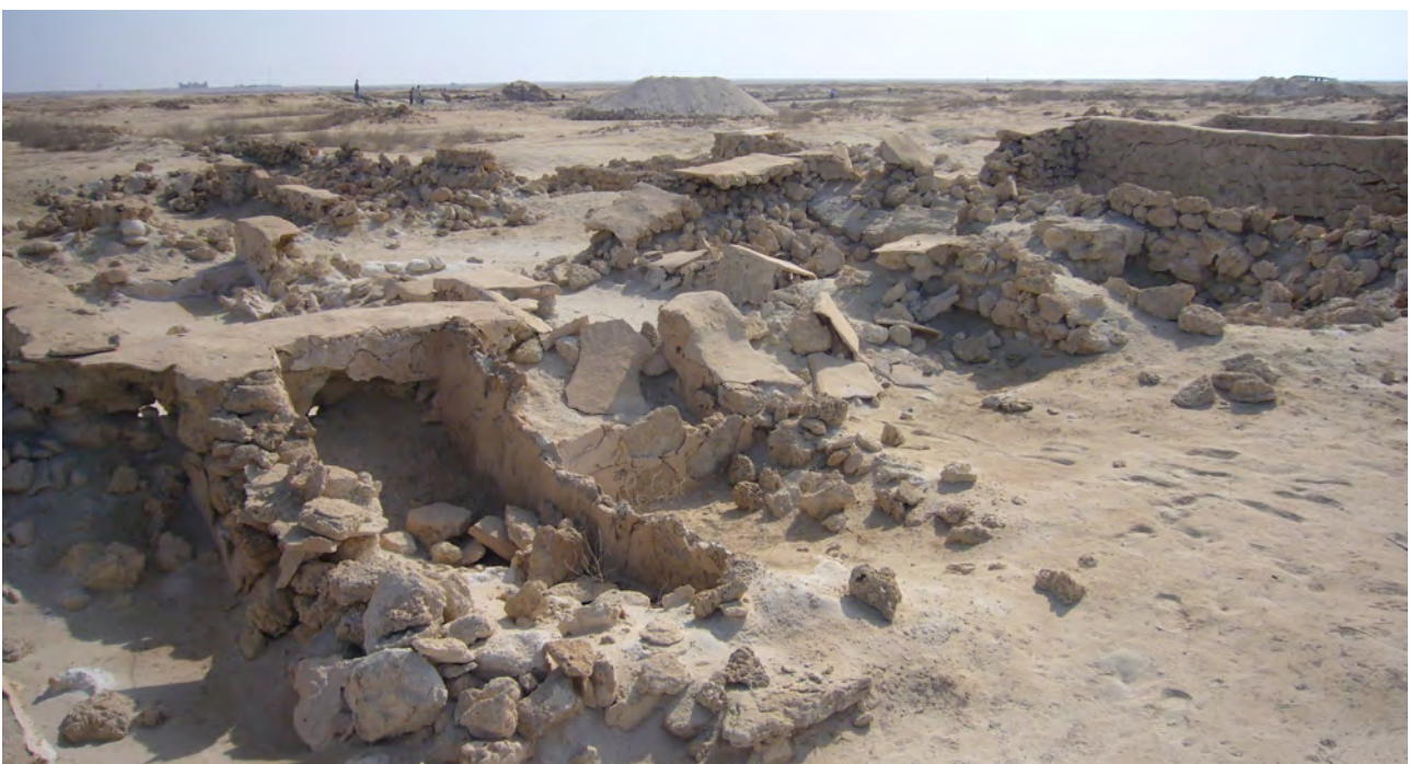
State of conservation of architectural remains restored in the 1980's in QMA1 (November 2009): Disintegration of building material; collapse of wall structures and cement capping.
