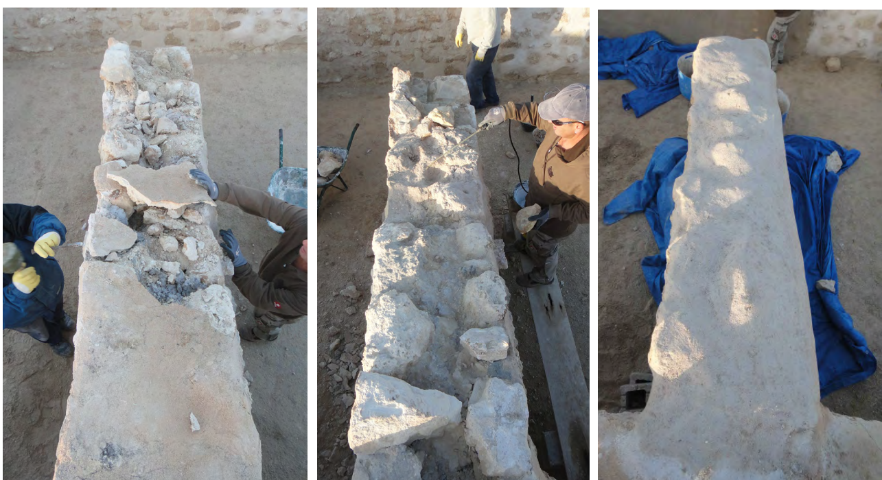
Consolidation of 1980s Restoration in QMA2: Taking off cement capping; Consolidation of wall structure, and re-shaping of wall top (2011/2012).
