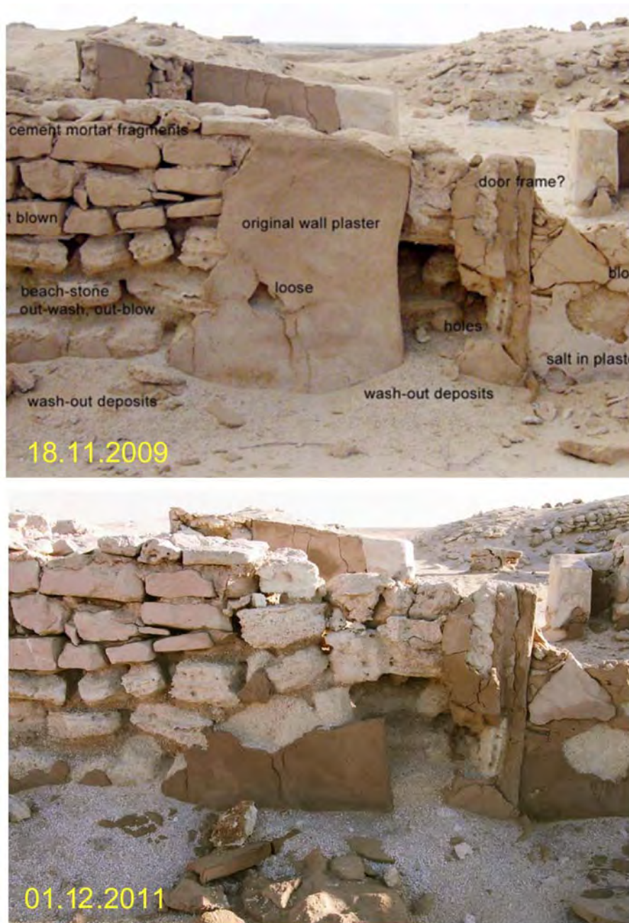
Figure 33: Loss of wall plaster at wall c, room 005, South Field
