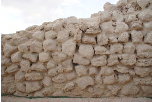
Open joints (e.g. ZUEP04, wall 4010)
