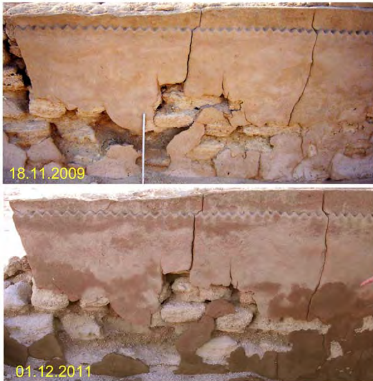
Figure 34: Loss of wall plaster at wall c, room 005, South Field
