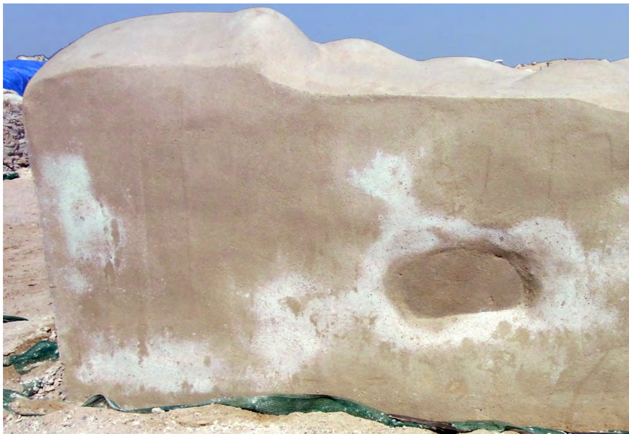
Fig. 1 b Crystallisation of sodium chloride (halite) on wall render at Al Zubarah.
