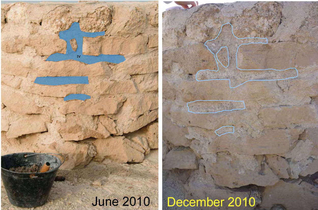
Figure 17: Test field IV with anhydrite mortar for jointing at NE corner of tower structure (Roman numeral refers to sample number in table 8)
