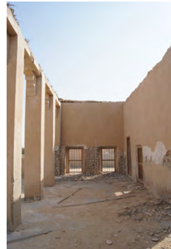
Al Jumail, S40 - mosque. Fragments of plaster, stones, blown-in sand deposits and litter visible on the floor
