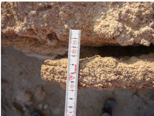
Poor bonding of plaster to wall structure (e.g. QMA4:5c)
