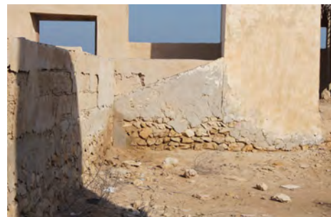
Al Jumail, mosque (S40). Masonry of cement blocks and stonework covered by cement plastering (left); the abluion room's wall has an additional layer of anhydrite finish (right)
