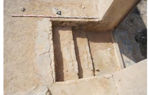
Al Jumail, S40 - mosque. Cracks on the steps leading to the courtyard of the mosque
