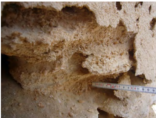
Voids in wall structures (e.g. QMA 4:4b)
