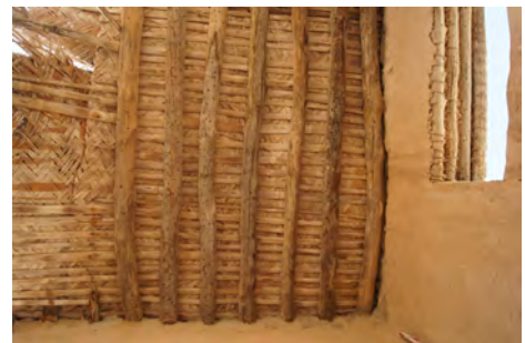
Al Jumail, S40, Roof of round beams, bamboo, woven mats and mud covering
