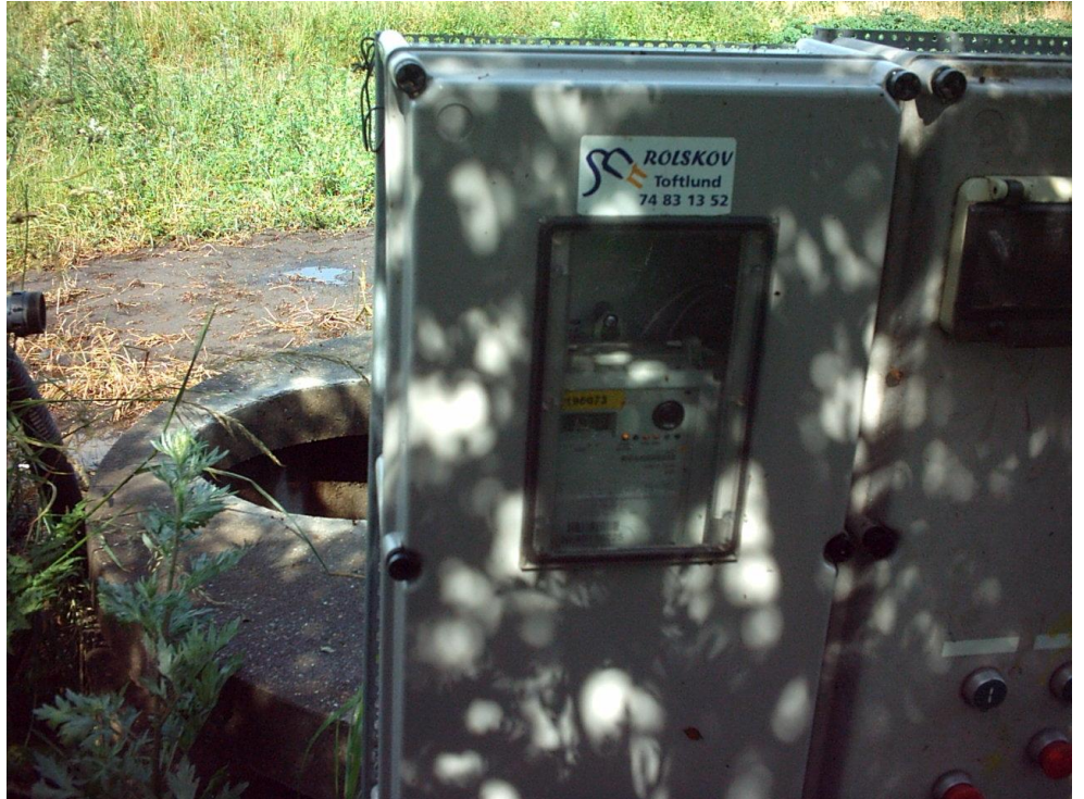
Photo 3 Field site well, meter (kWh and hours), and control unit
