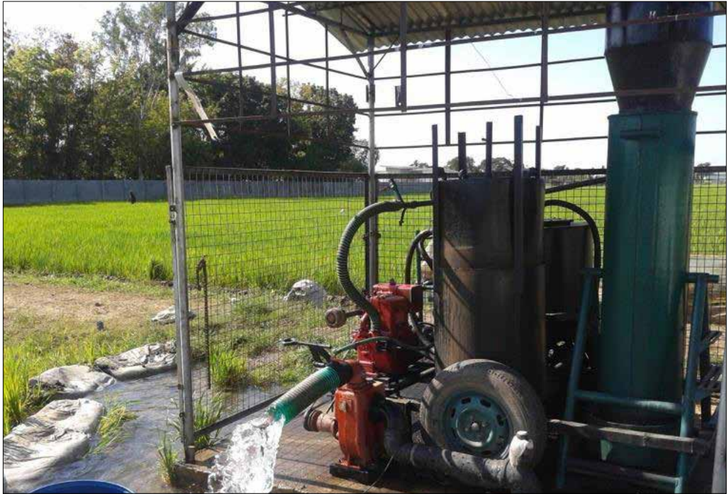
Figure 2.29. An example of a shallow tube well pump
