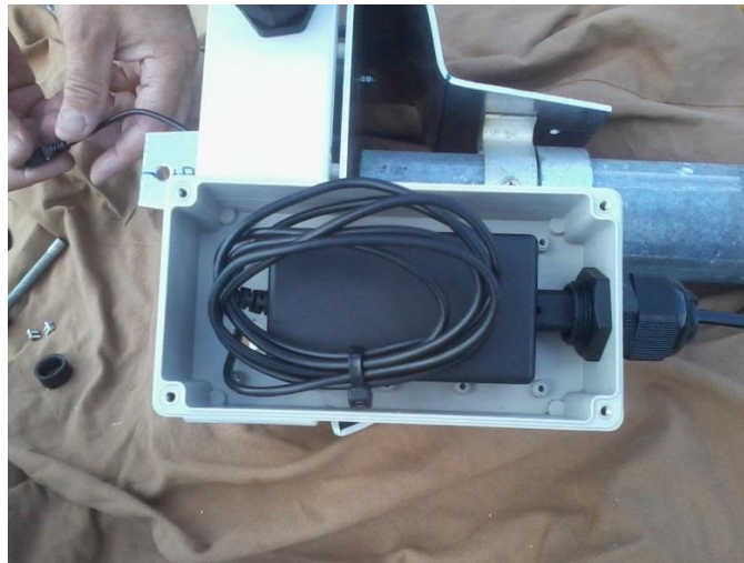
Figure B.1 – View of the compartment enclosing the power supply of the camera.
