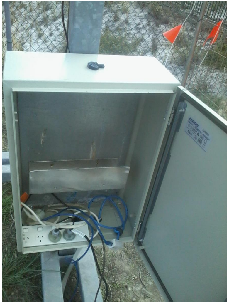
Figure B.4 – View of the cabinet containing the computer and the hard drive.
