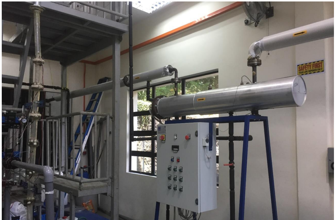
Figure 3.4: Superheater installed along the steam pipeline
