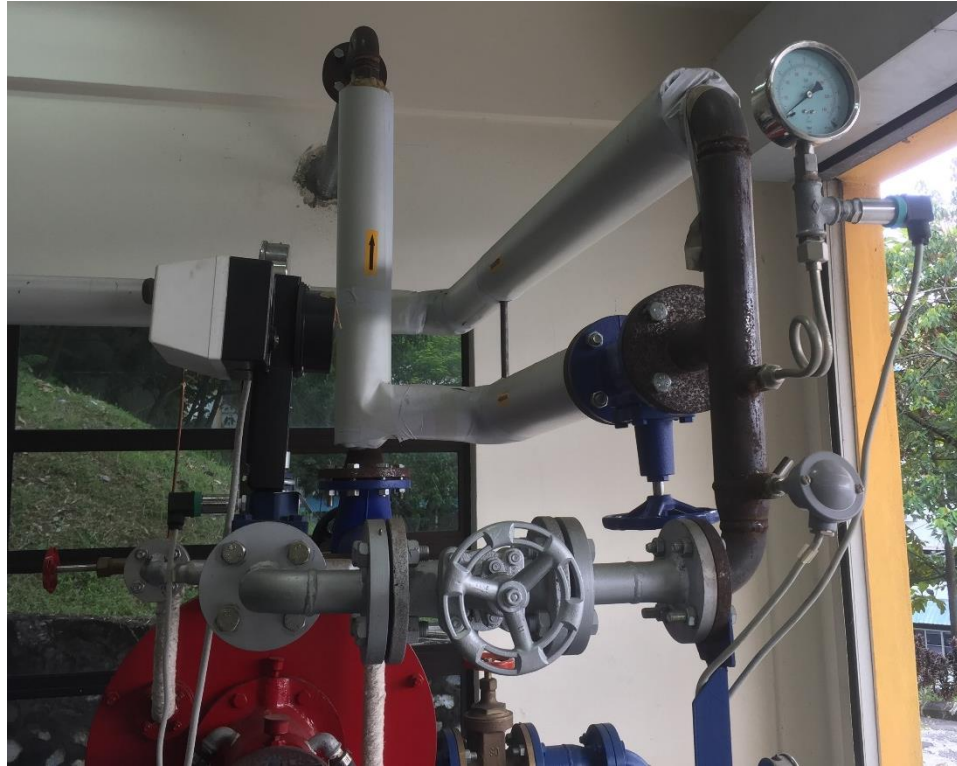
Figure 3.5: Pressure gauge, P_2 connected at turbine
