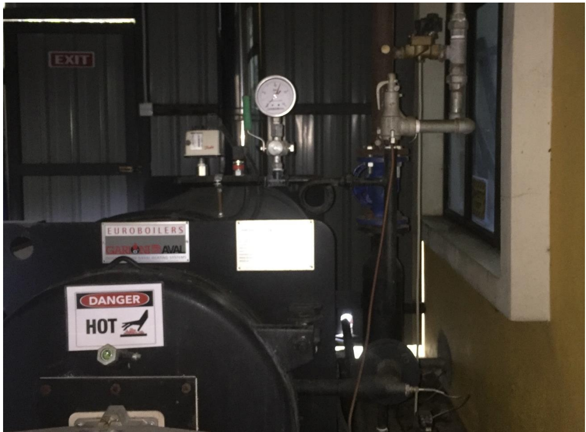
Figure 3.3: Pressure gauge, P_1 connected at boiler
