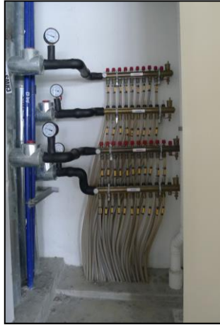
Figure 4.10: Chilled water pipes for floor slab cooling system
