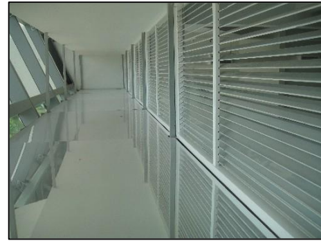
Figure 4.7: Mirror light shelf and fixed blinds installed above windows (Source: Mohd Yusof, 2012)
