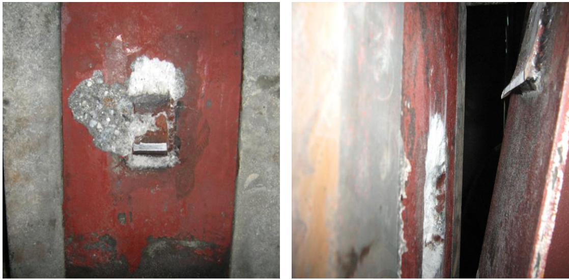
a) Fractured channel in slab
