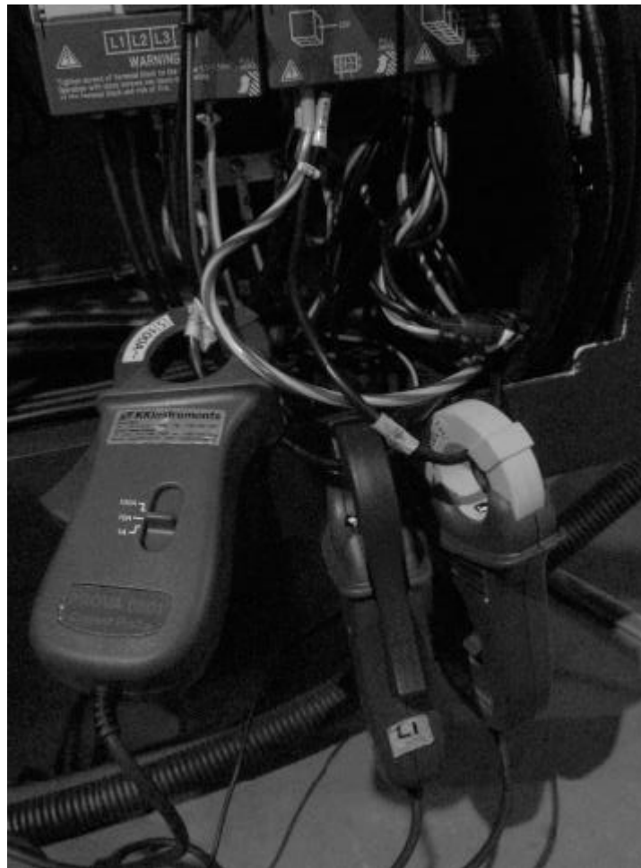
Current and Voltage probes connected to the servo motors and spindle motors connection in the PLC
