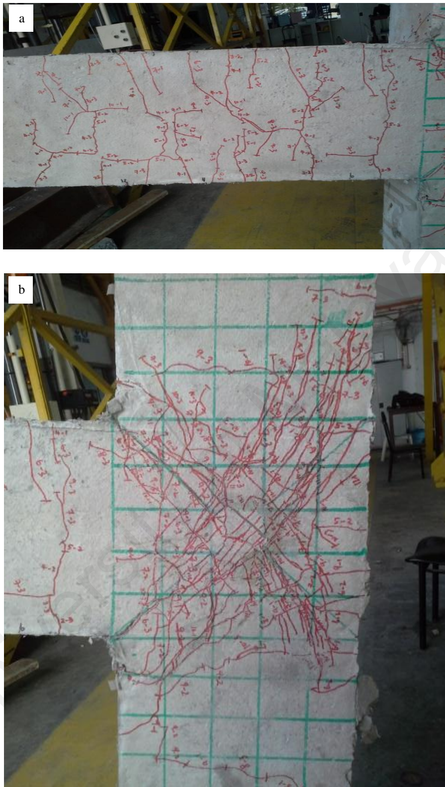
Figure 4.38 Crack propagation in (a) beam (b) joint zone of PE 3 beam-column specimen
