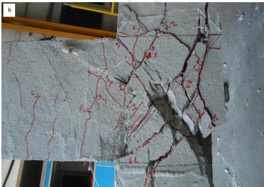
Figure 4.28: Crack propagation in (a) beam (b) joint zone of the NC 1 beam–column specimen
