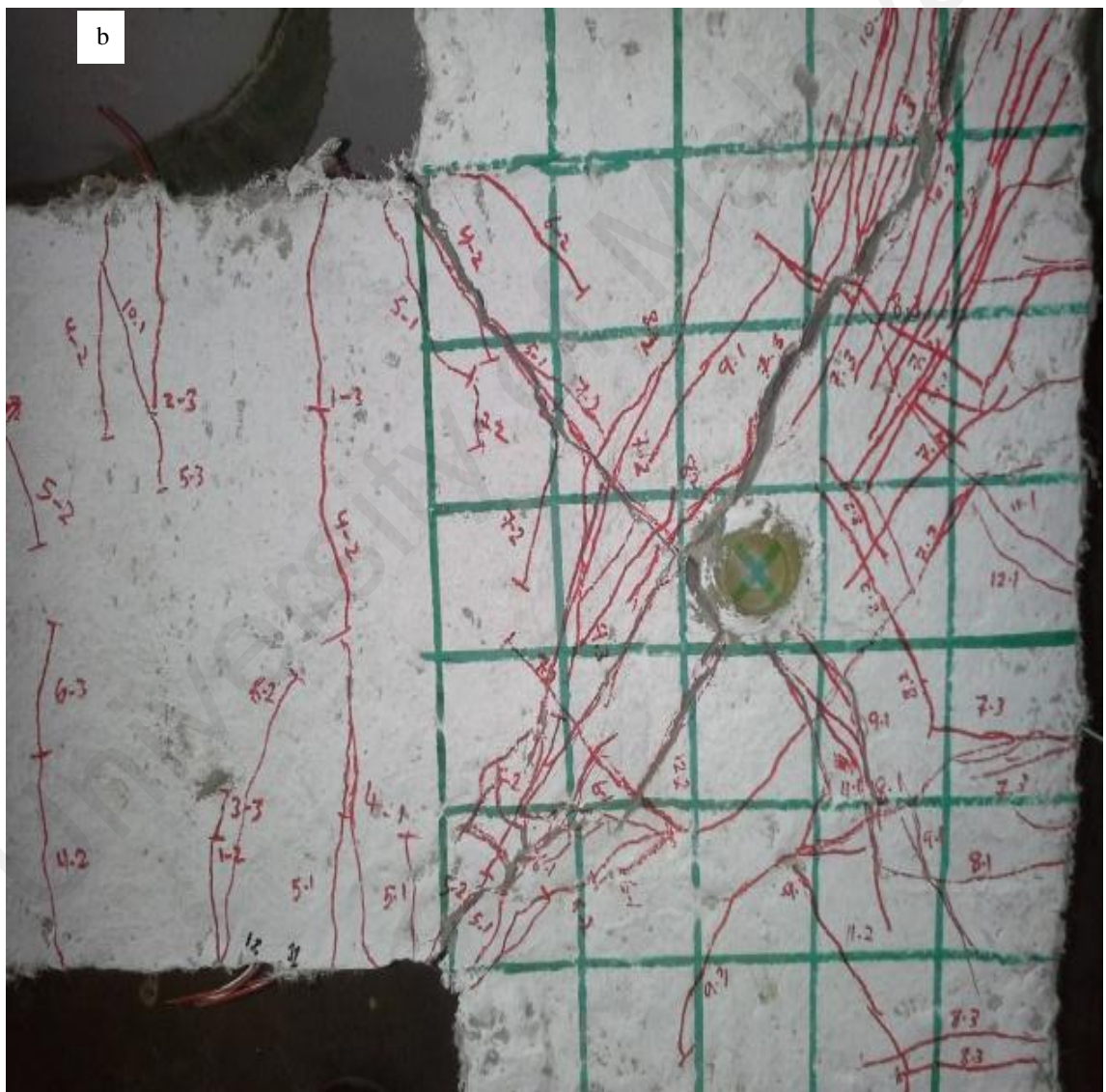
Figure 4.32: Crack propagation in (a) beam (b) joint zone of PVA 3 beam–column specimen
