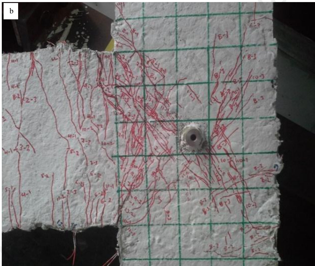
Figure 4.36 Crack propagation in (a) beam (b) joint zone of PE 1 beam–column specimen
