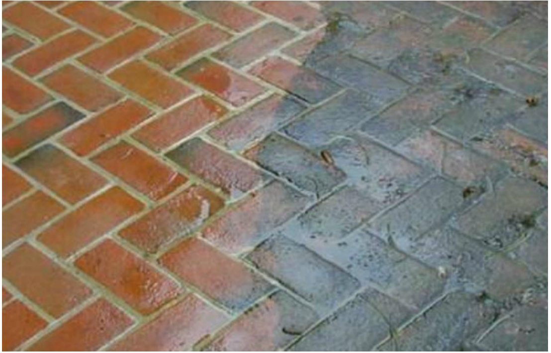
Figure 4-2: Example for Bad Floors in Restaurants
