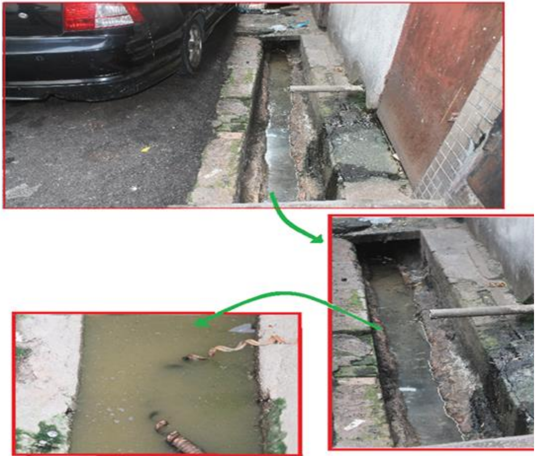
Figure 4-4: Example for Bad Drains in Restaurants; the images from multisided of the drain
