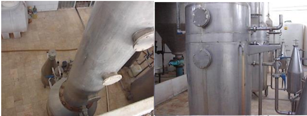
APPENDIX E4: Condenser (cooling tank)
