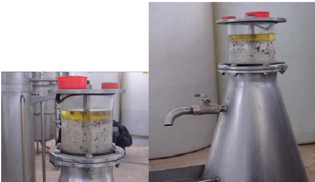
APPENDIX E5: Oil separator tank (essence pitcher)
