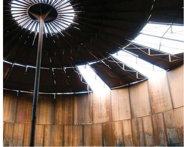
FIGURE 5. Interior of an abandoned silo Ruriksson, B. (Photographer). (2007). Inside a Steel oil tank [digital image]. Retrieved October 1, 2014 from http://trivoxphoto.photoshelter.com/image/I0000oRsS_5dF3kQ
