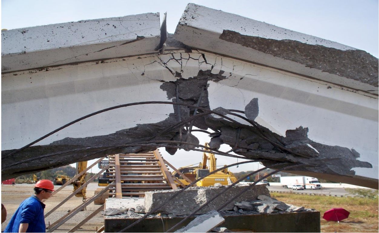
Figure 31. Prestressed beam after impact.
