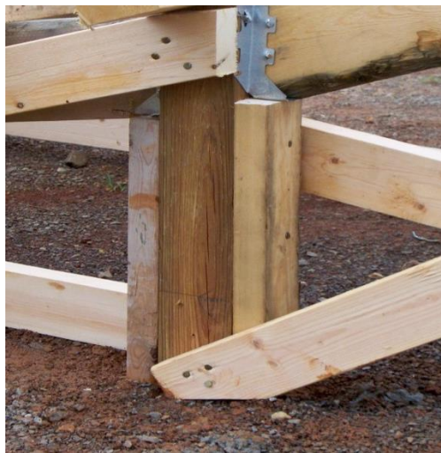
Figure 19. Added 2x4's for extra compression reinforcement.
