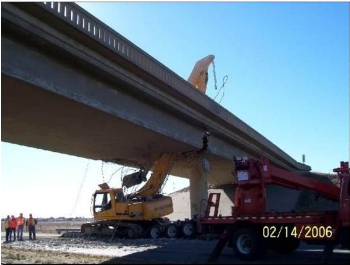
Figure 2. Damage caused by overhead collision. (DailyCognition, 2013)
