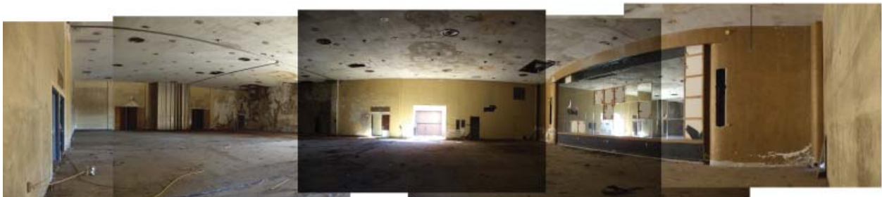
Figure 33. Between the Hotel and the Annex: the ballroom. Sources: Photographs and montage by author.
