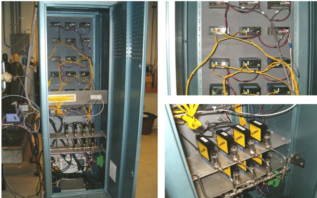
Figure 3.23: Photograph of the back panel of the instrumentation cabinet.
