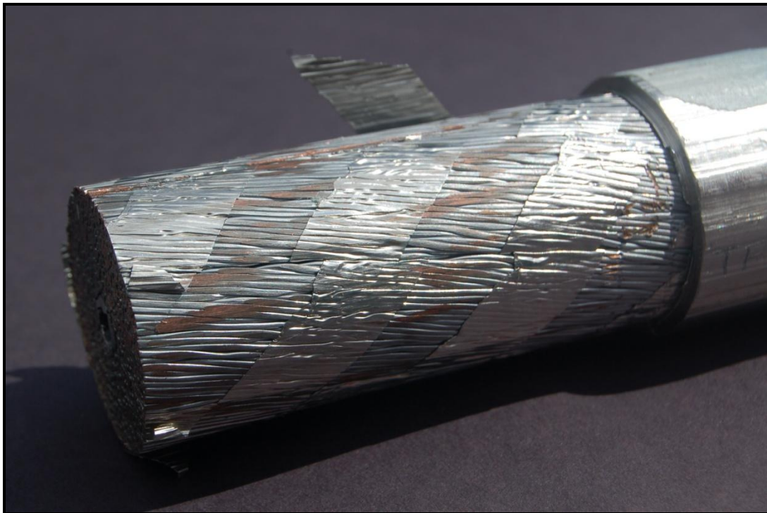
Figure 4.14: TF-WC1 Copper Cable Exposure from grip sleeve slippage
