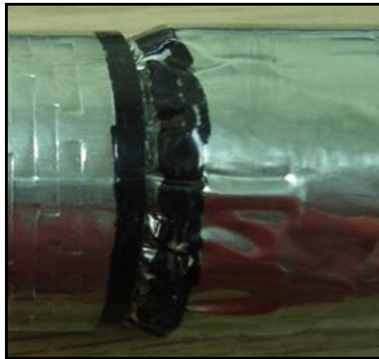
Figure 4.99: Lack of foil wrap folding due to lack of cable rotation
