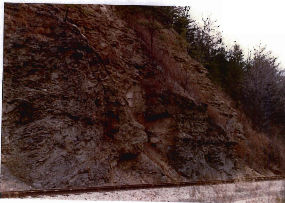
Figure 14. Parallel fractures at Field Station 55.
