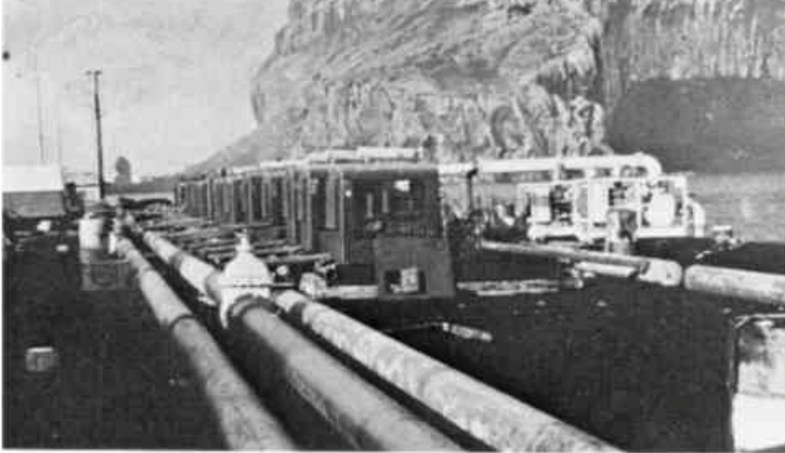
Figure 1.08 Seawater Pumping System On the Coast Source: http://pubs.usgs.gov/of/1997/of97-724/water.html
