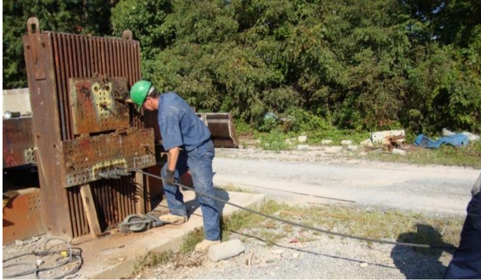
Figure 52 Laying of 0.7 in. strand through the dead end of the prestressing bed
