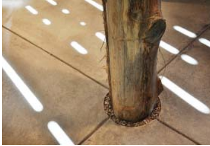
Figure 38: Column Base Detail. Yew Dell Botanical Gardens. DeLeon and Primmer Architectural Workshop
