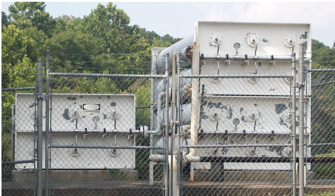
Figure 23. Outdoor Tank Farm of 18 High Pressure Cylinders
