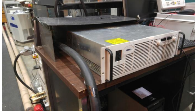
Figure 35: Power supply with plastic enclosure to prevent shock hazard.
