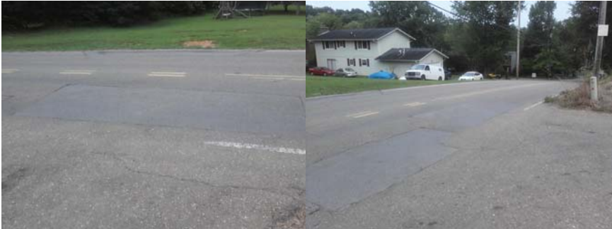
Figure 193 – Photographs – 1512 Andes Road, WKUD
