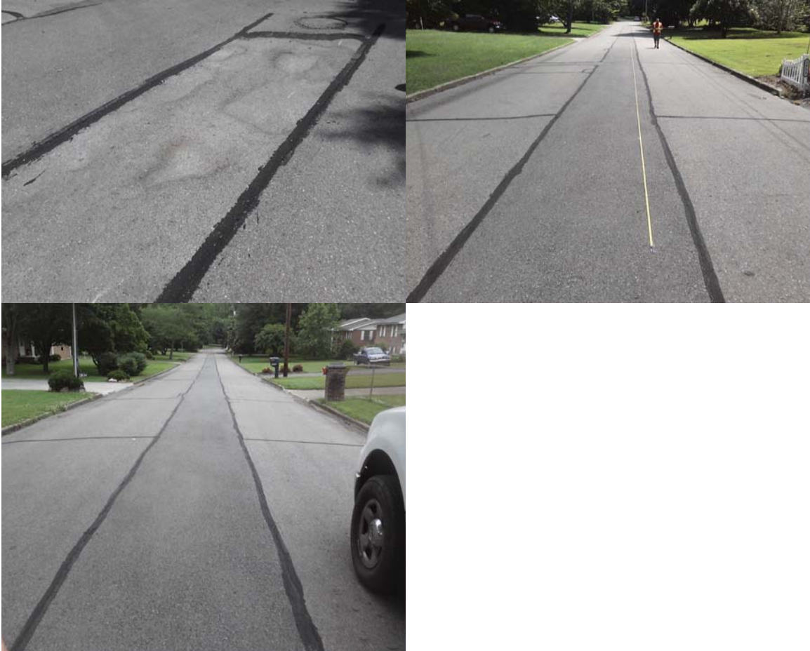
Figure 49 – Photographs – 1834 Timbercrest Drive, AUB
