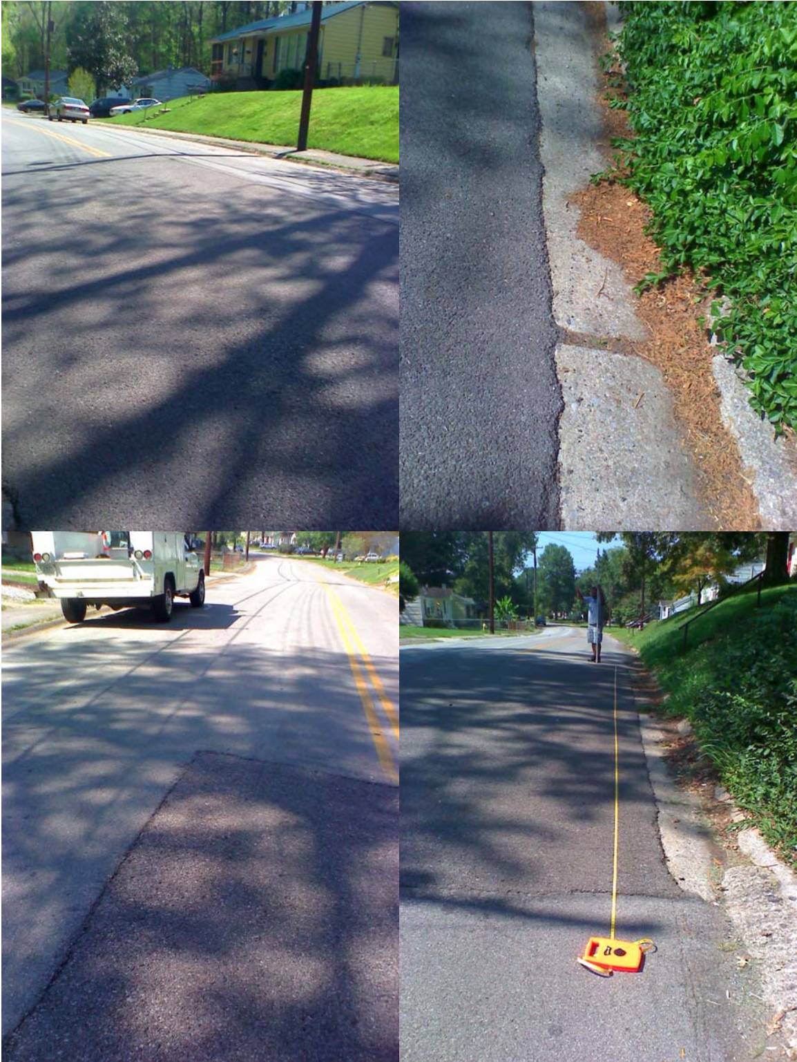
Figure 106 – Photographs – 237 East Drive, COR
