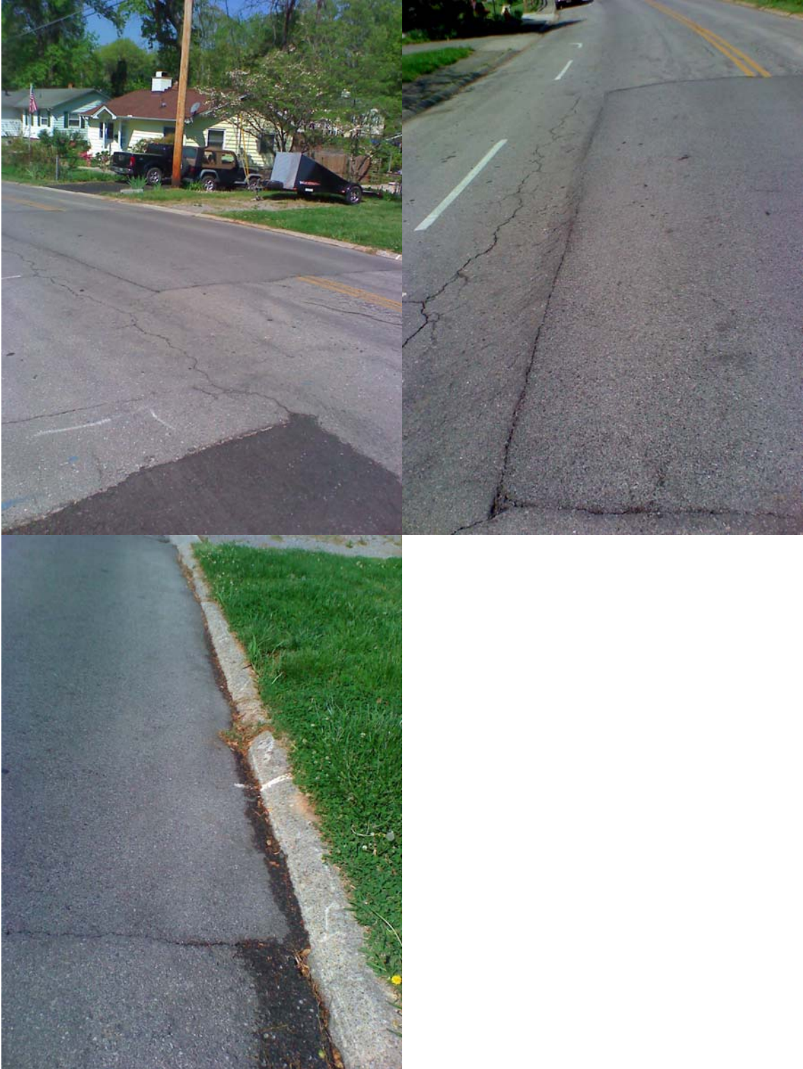
Figure 110 – Photographs – 440 East Drive, COR
