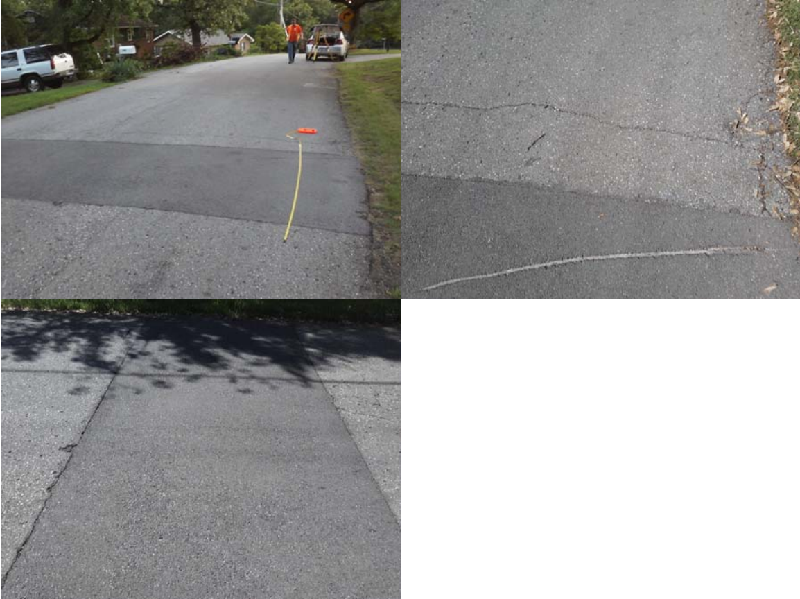
Figure 79 – Photographs – 1140 View Drive, COM
