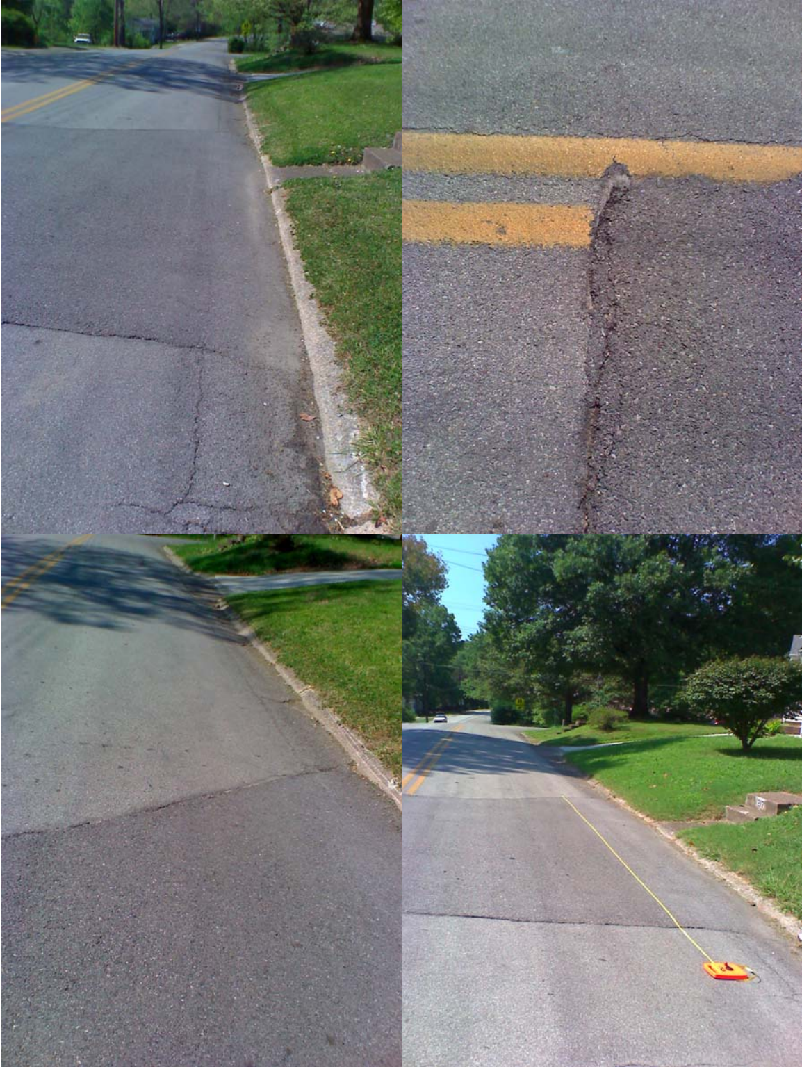
Figure 103 – Photographs – 217 East Drive, COR
