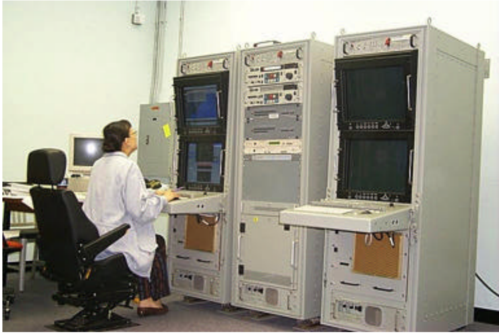
Figure 2-5. Tactical Control Station Operators Station
