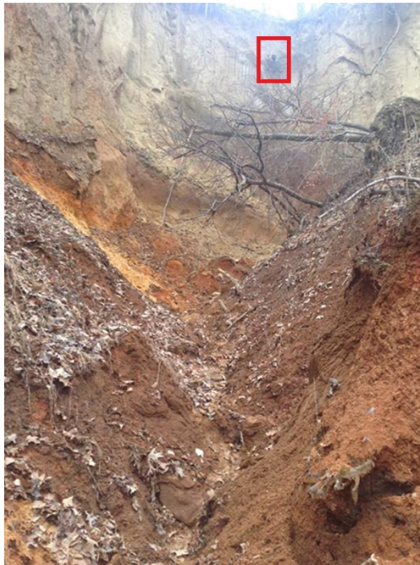
Figure 5. Photograph of the pool gully channel. The drainage pipe is visible inside the red box at the top of the photograph.
