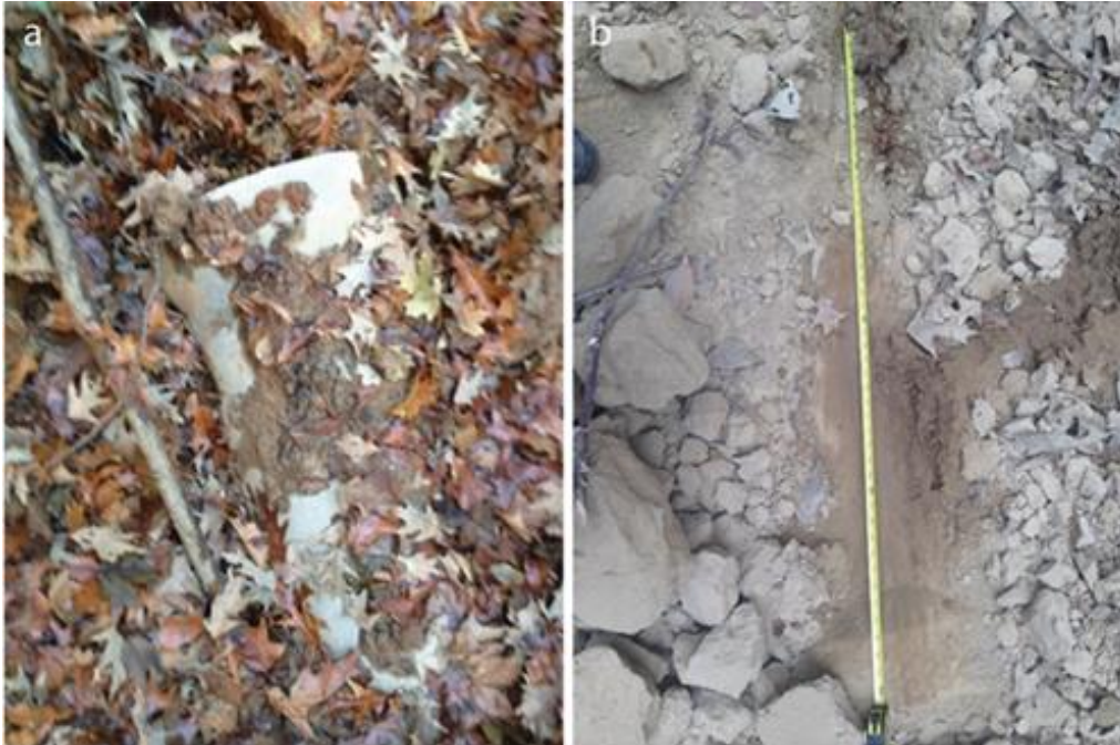
Figure A2. The photographs were taken near the base of the gully headwall on (a) 12/24/2014 and (b) 02/08/2015. A section of the pool drainage pipe is shown to have fallen and been buried by material from the headwall.
