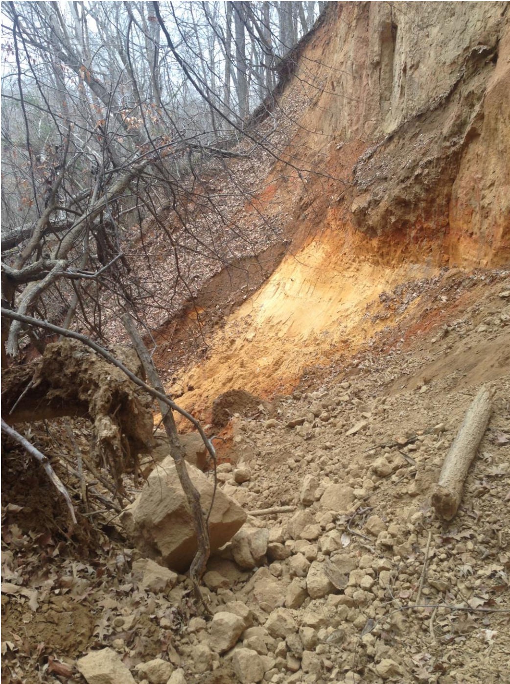
Figure A1. Headwall material deposited in the gully channel
