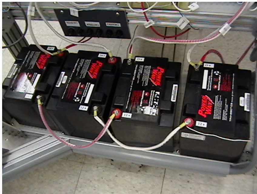
Figure 6.2 Actual batteries connection
