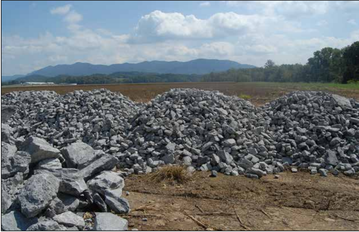
Figure 3.6 –Rock and stone used for filling sinkhole.
