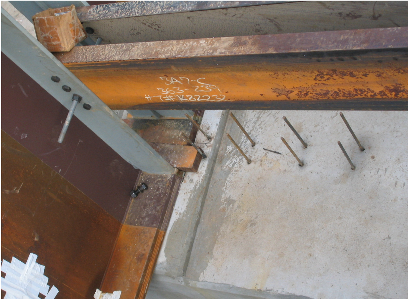
Figure A33: Photograph of Kicker Wedge Plates, Girders, and Diaphragm Reinforcing Steel (Kicker Wedge Plate installation is not complete)
