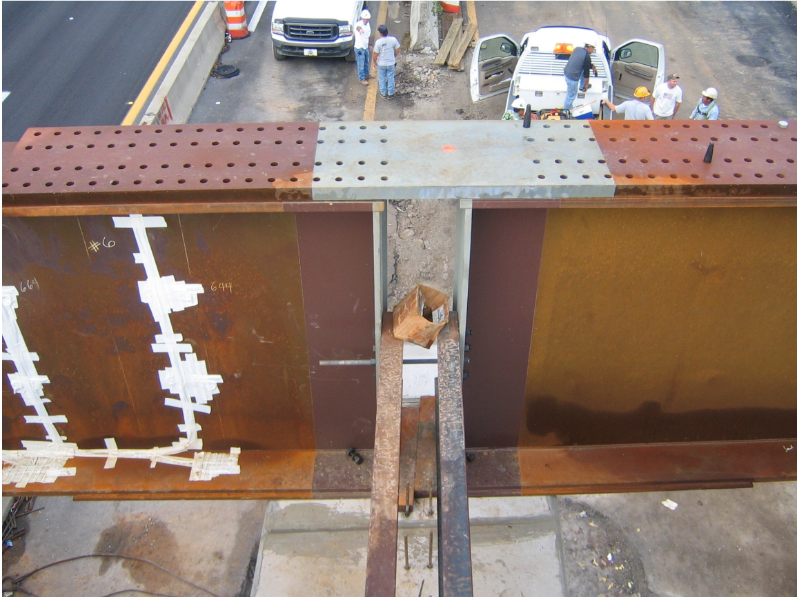
Figure A10: Photograph of Connection Before Bolt Installation (View looking west at Girder 6 from Girder 5)
