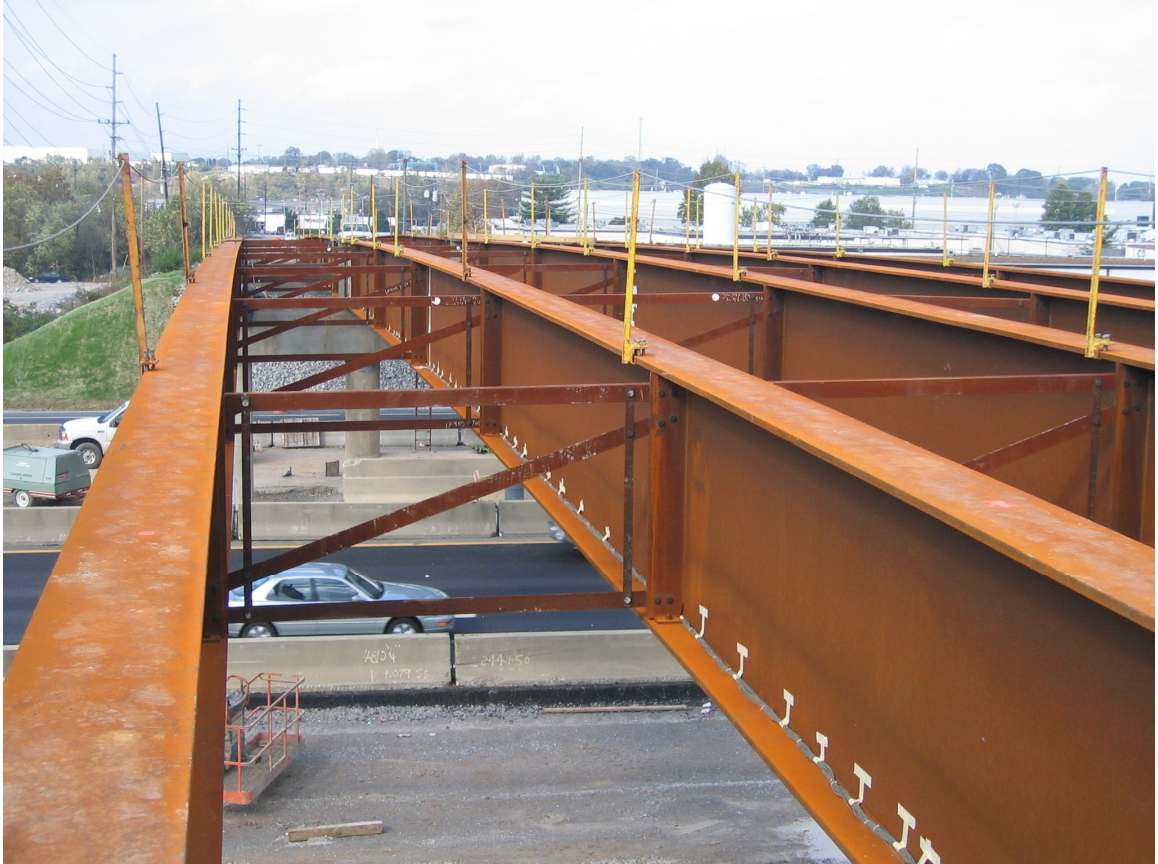
Figure A9: Photograph of Girders After Being Erected (View from the South Abutment)
