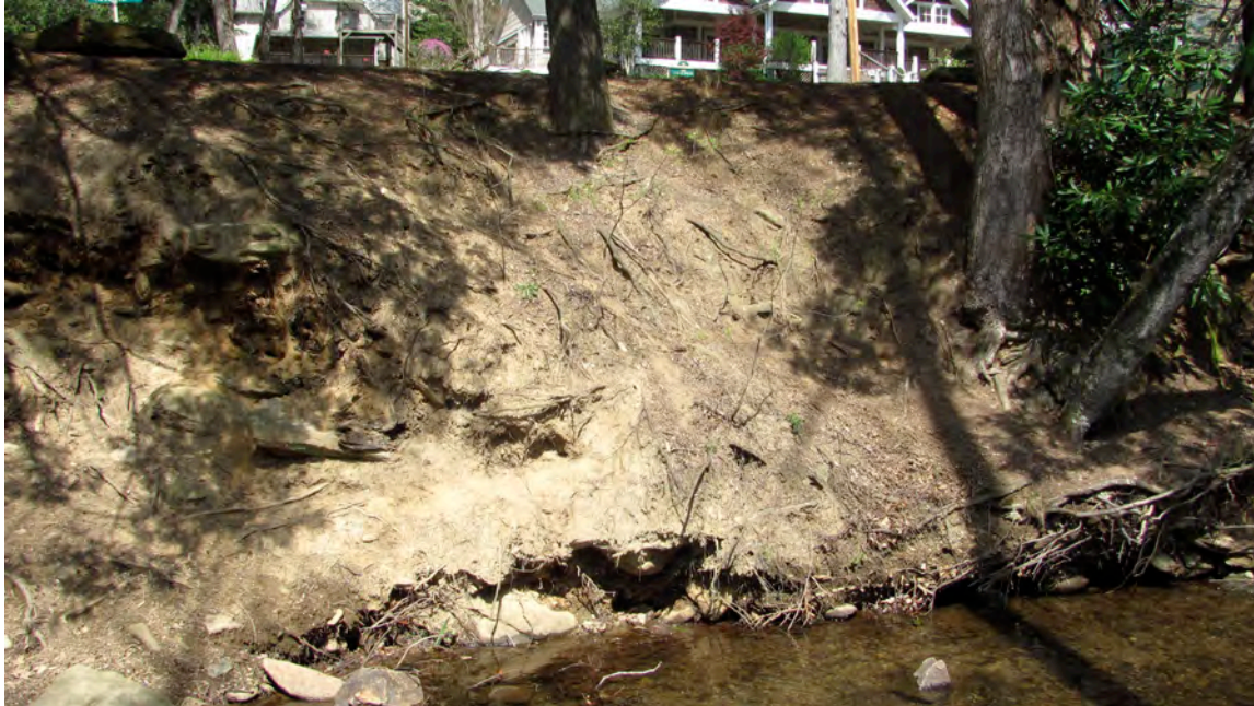
Figure 4.4 - Eroded riparian zone along Flat Creek in downtown Montreat*
