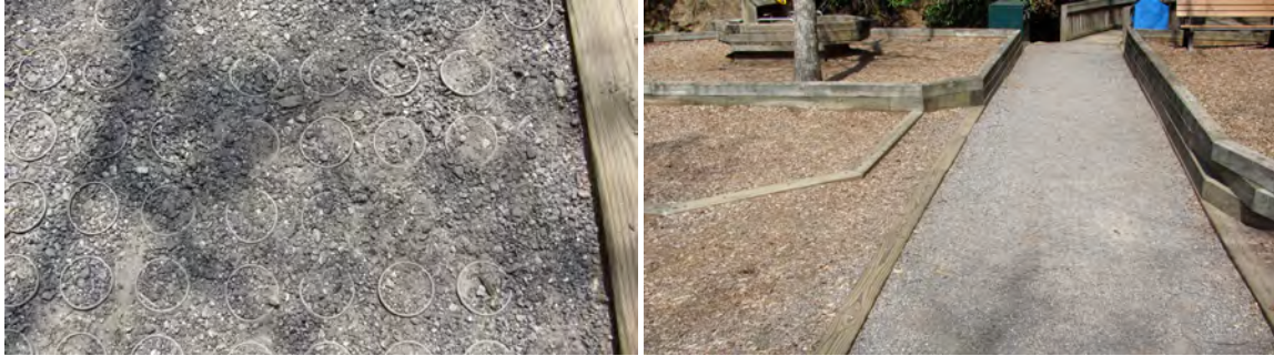
Figures 3.3 & 3.4 - Permeable pavement system in a park in downtown Montreat*
