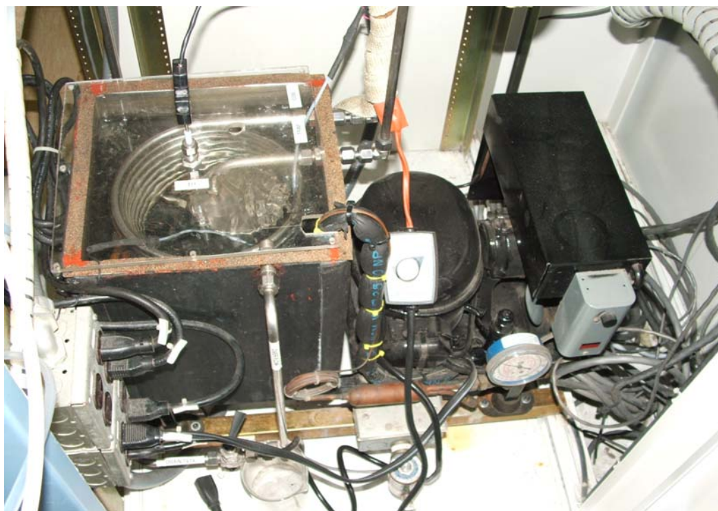
Figure 3.11. Water Condenser Inside of the Horiba Analyzer Bench.
