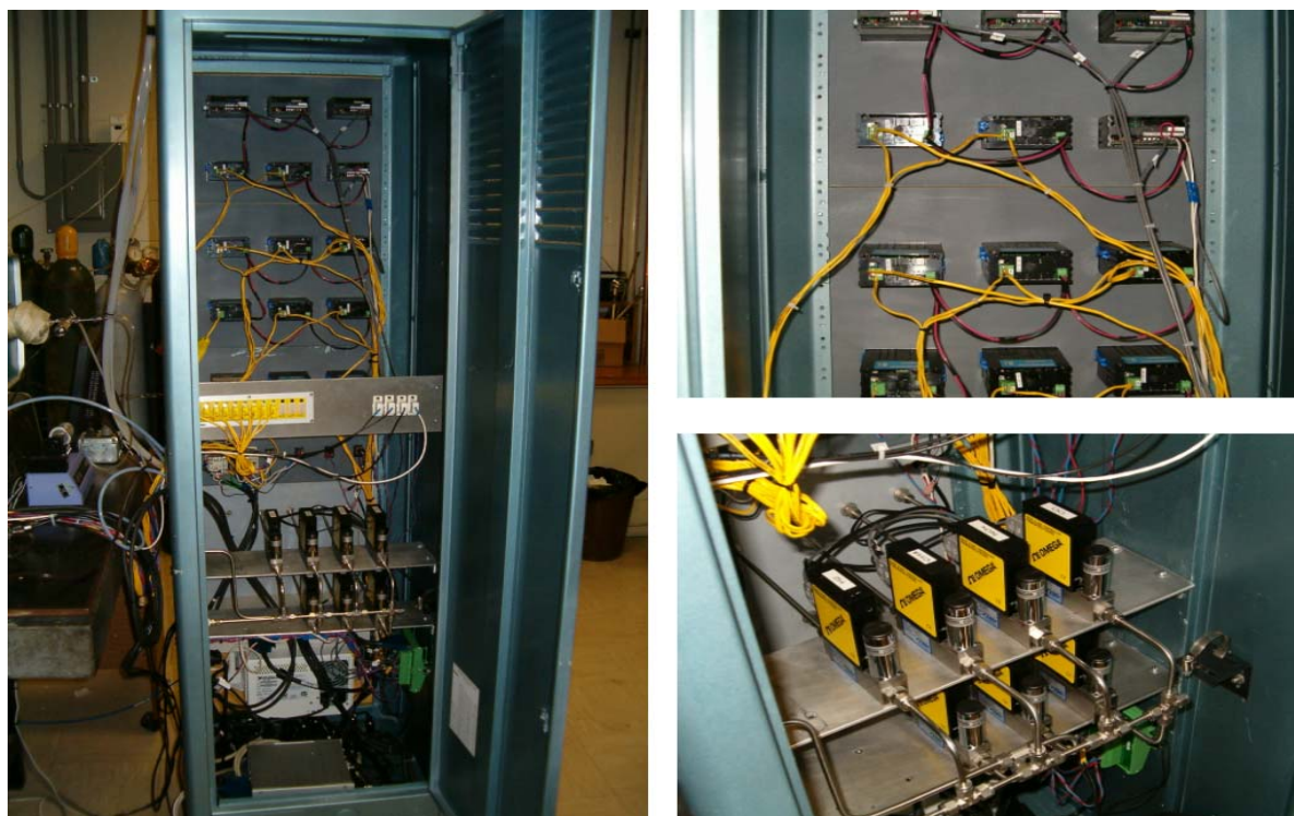
Figure 3.15. Wiring of Displays and MFC Inside the Instrument Cabinet.
