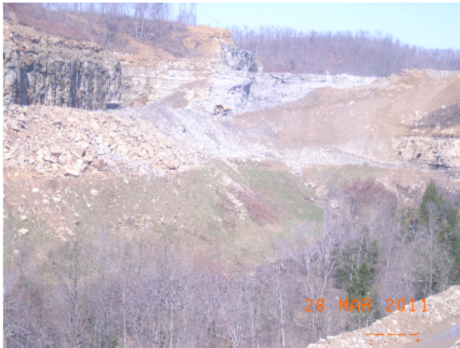
Figure 26: Site Photo B - Rock (spoil) material is being hauled from the left side of the photo to a reclamation site located on the right of the photo (Curry).
