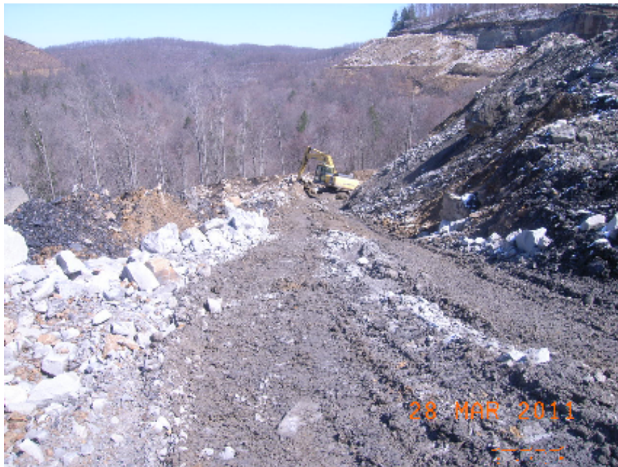
Figure 30: Site Photo F - A Hoe (Excavator) doing "Self-Recovery" with a thrown track. The right side track came off and the operator is carrying the track and traversing the cab/boom to crawl back up the ditch on the good track to some level ground (Curry).
