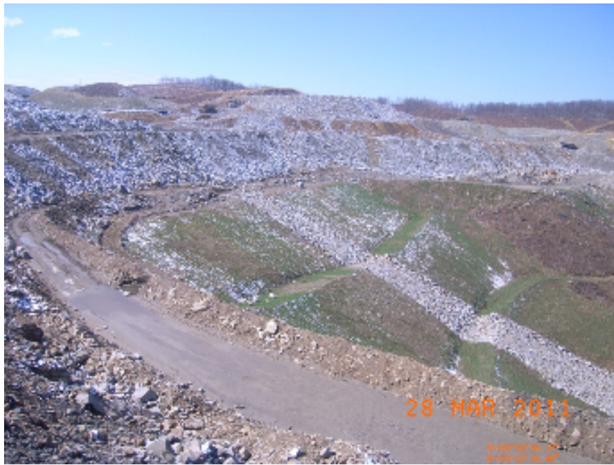
Figure 29: Site Photo E - The trucks are Caterpillar 777's, the tires are 20' tall. The black pile on upper left is a coal stockpile (Curry).
