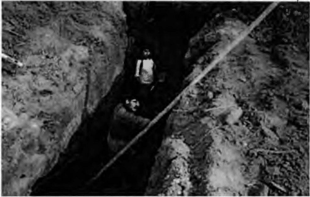
Figure 8 – Example of a Trench without Protection
