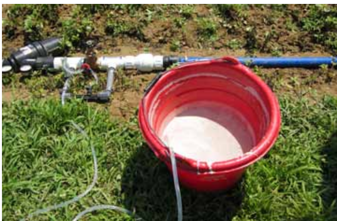
Check Valve, Injector, Screen Filter, and Batch Tank for Fertigation
