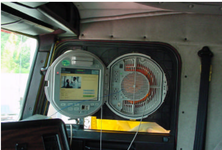
Figure 1.3. IdleAire in-cab HVAC module and computer terminal.
