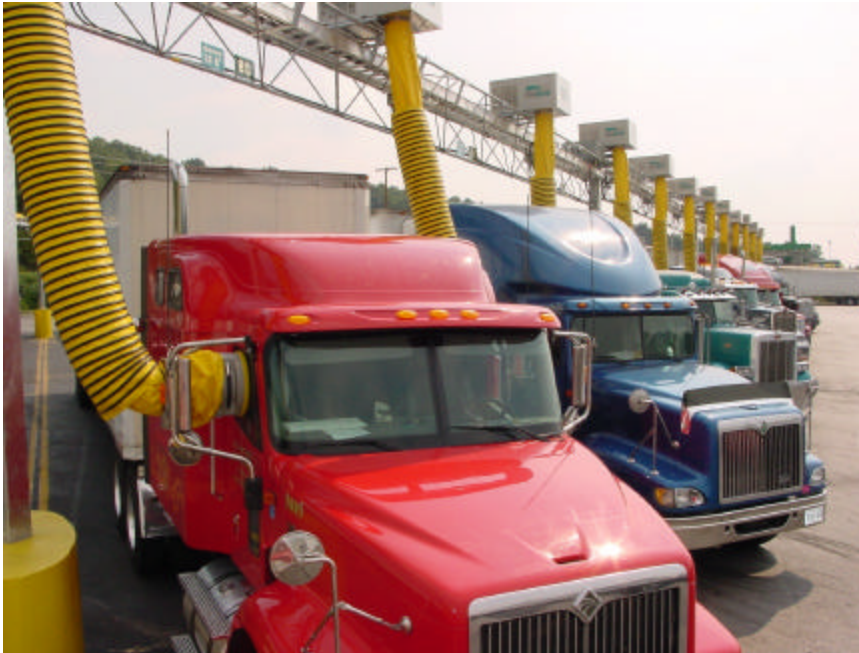
Figure 1.2. Truck stop electrification at parking lot (rest) area.
