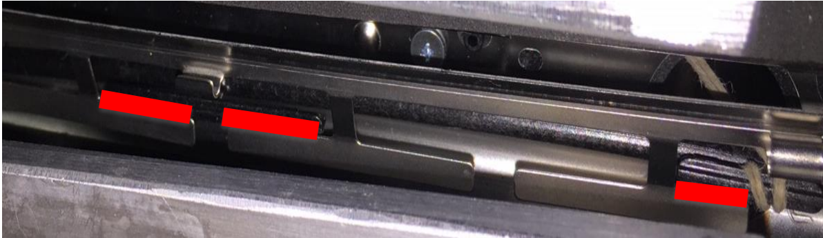
Figure 10. Additional Problem: Interference with Metal “T’s” Due to Extreme Deflection of Agitator Shaft (Marked by Red Zones)
