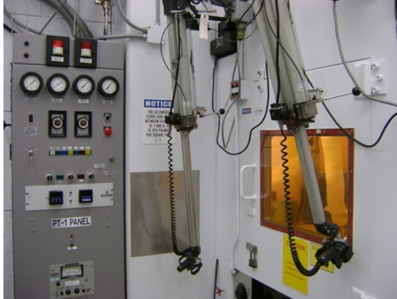
Figure 4.5: PT-1 Facility with Shielded Cubicle
