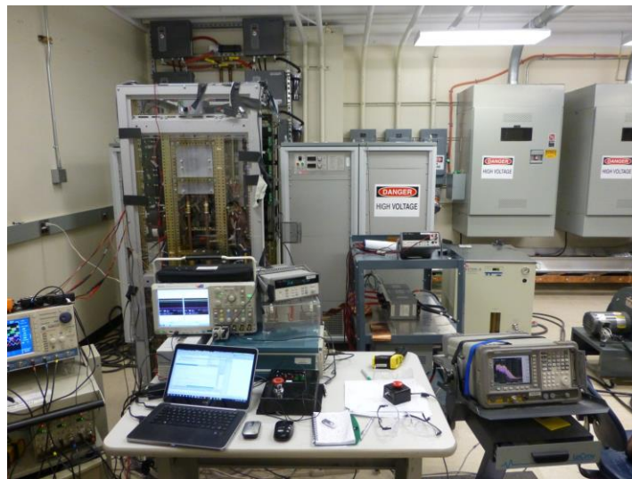
Figure 7.31. 100 kW motor drive system test setup
