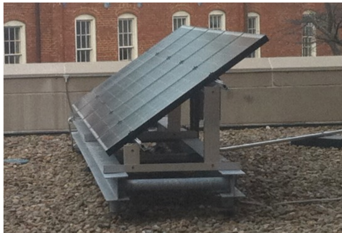
(a) Solar panels Sanyo HIP-195BA19
