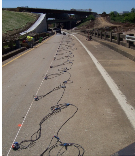
Figure 2.6. An array of Geophones installed on the bridge deck over the center beam
