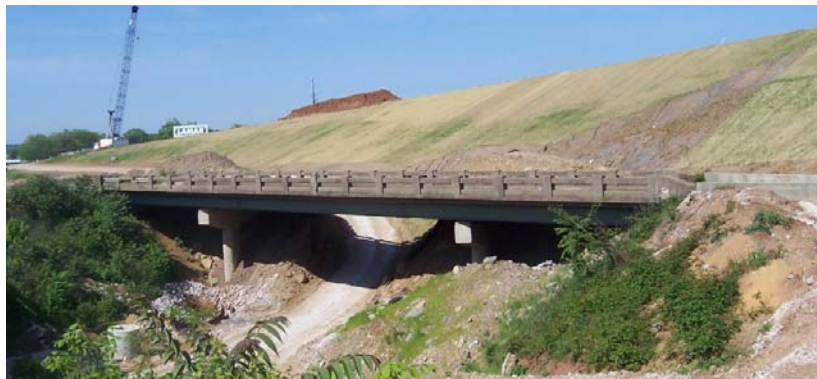
Figure 2.4. Photo of the entrance ramp to James White Parkway from I-40 westbound
