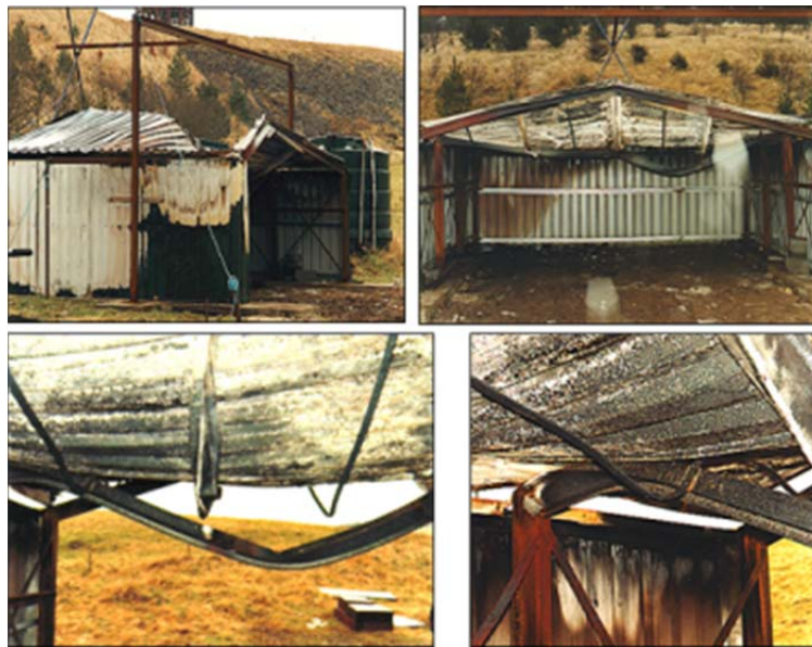
Figure 2.7: Deflection and failure of portal frame building (Wong, 2001).
