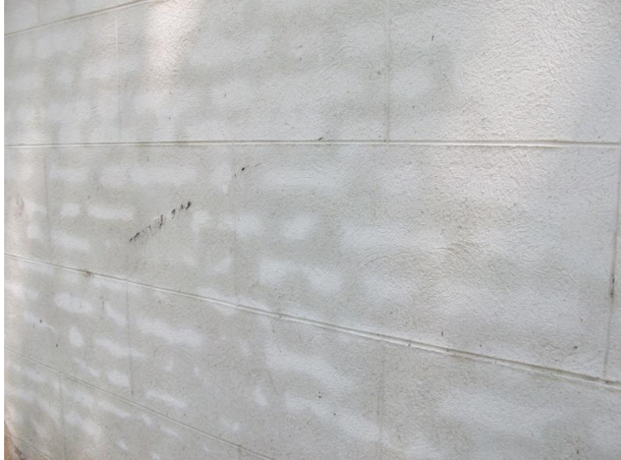
Figure 3-15. Exterior wall of Strawberry Chapel. While the outer surface is stucco carved to give the appearance of stone, the brick pattern underneath the stucco can clearly be seen due to the underlying mortar holding in moisture (Photo by the author).
