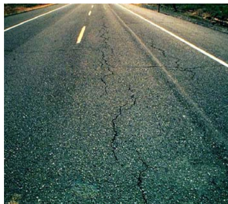
(b) Longitudinal cracking (wheel path)
