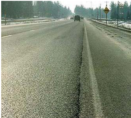
(c) Longitudinal cracking (non-wheel path)
