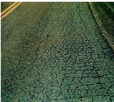
(a) Alligator cracking
