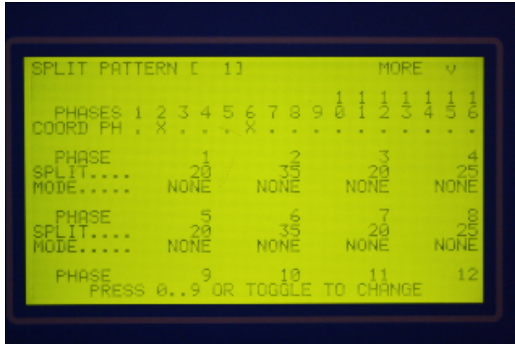
Figure 3 - ASC/3 controller application of the common initial signal timing
