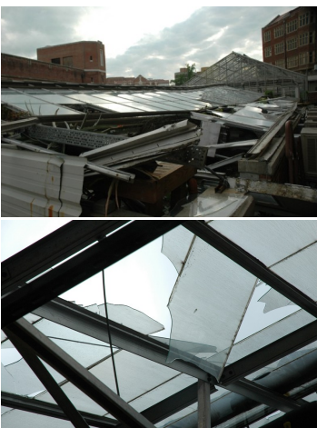
TOP: The freestanding greenhouse collapsed in strong winds on April 25.
