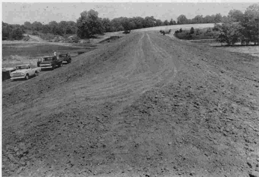
Structures, such as this newly-completed one on Sand Creek Watershed in Fayette County, hold back floodwater and gradually release it so as to prevent or reduce flooding below.
