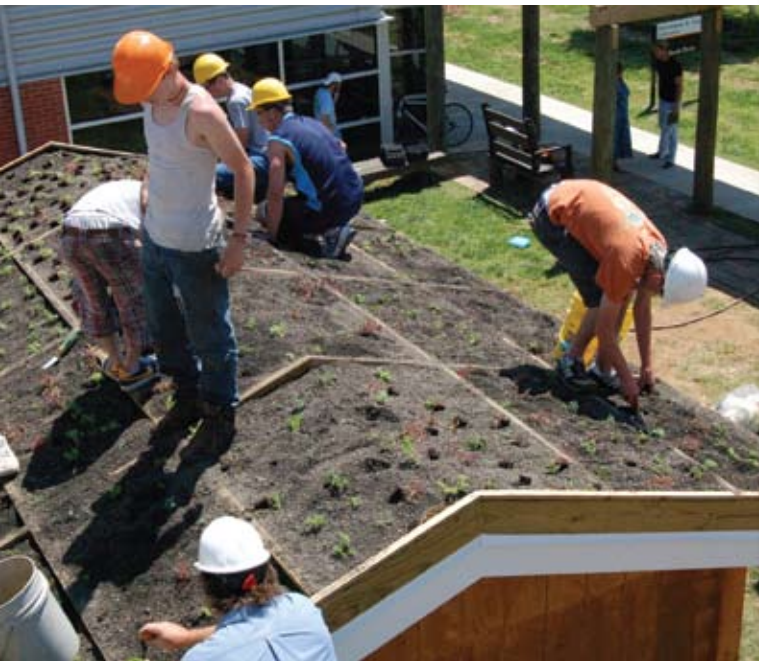
Students from the Byington-Solway Career and Technical Education Center assist in the installation of UT's first greenroof, adjacent to the Environmental Landscape Bldg. on the Ag Campus. This greenroof will aid in low impact development design and research as well as provide valuable information for the public. Photo by Curtis Stewart.
