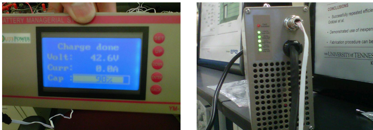
Figure 5.5. Charging complete as displayed by the BMS (Left) and charger (Right).
